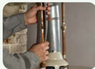
Water Heater Blanket and Pipe Wrap
